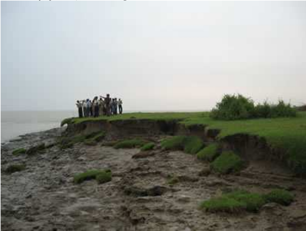
Fig.1. View of eastern flank of the Nayachar Island showing erosion. GSI team accompanied by officials from West Bengal Government carrying out investigation.
